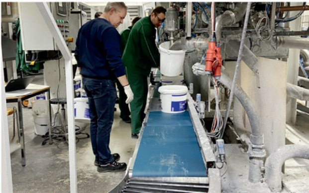
The weight controller Maxxis 5 regulates the filling system control unit automatically.
